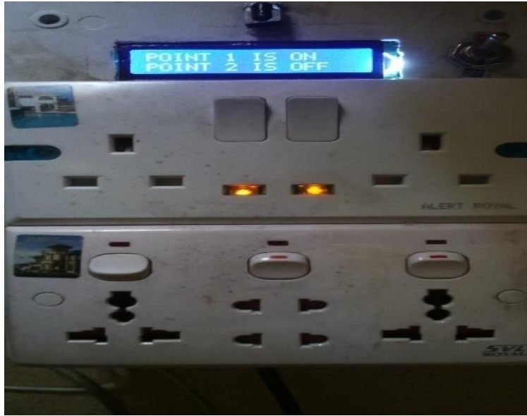
Figure 5: Point 1 ON and Point 2 OFF
